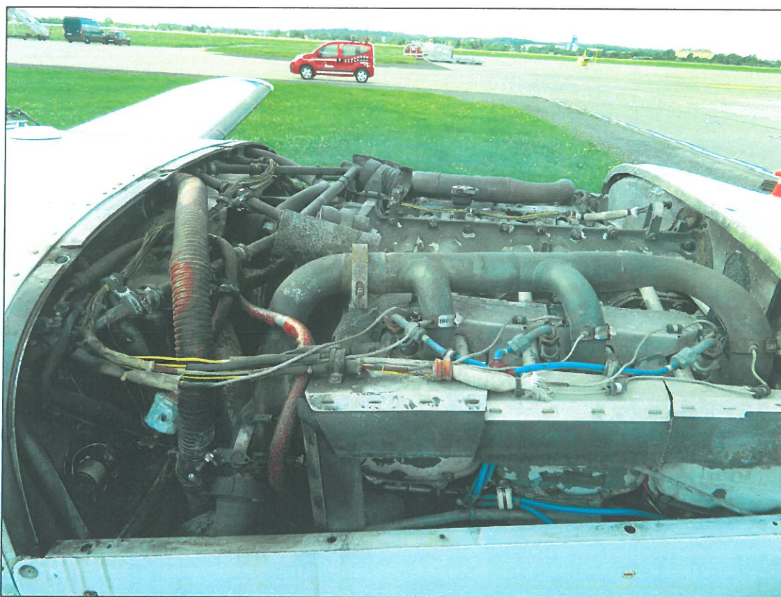
Fig.1. Damage to the engine compartment – general view
