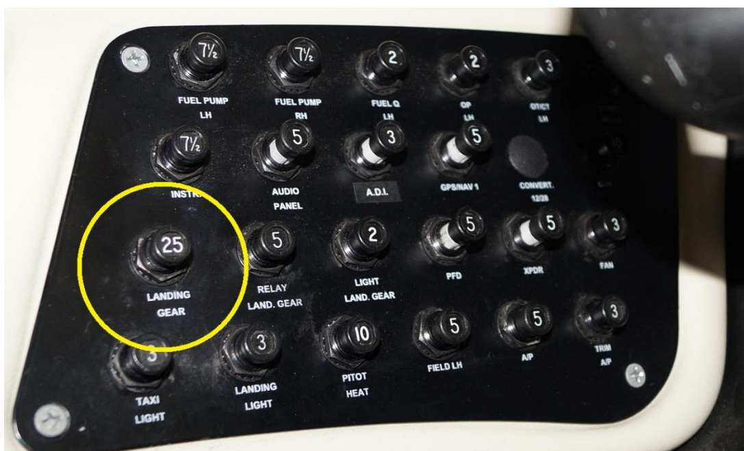
Fig. 10. The circuit breakers panel of the Tecnam P2006T aircraft with the marked “LANDING GEAR” circuit breaker
