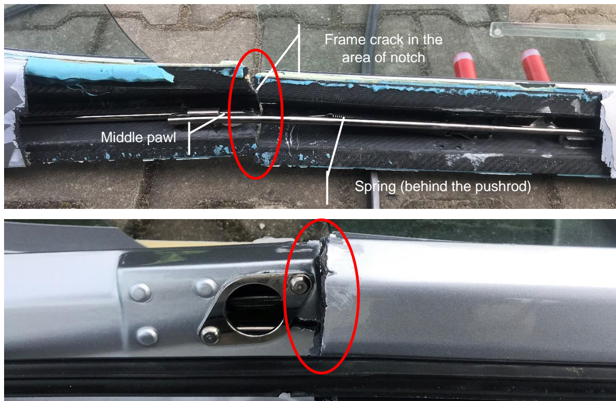
Fig. 8 Cracked canopy frame in the area of middle pawl location. A notch is present on the edge of fitting slot reinforcement [source: SCAA]
