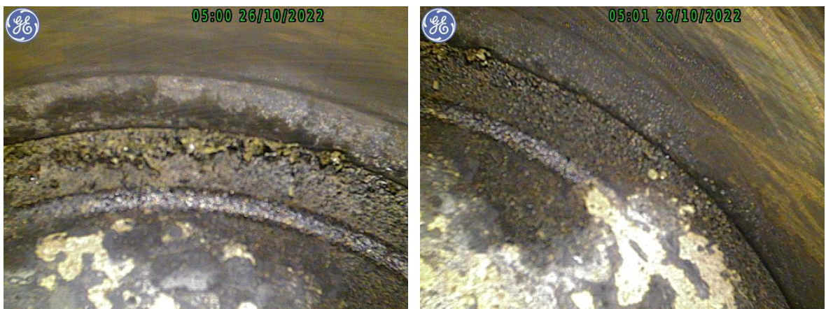
Fig. 15. Internal corrosion of the cylinder no. 1. Pictures were taken with the borescope camera [source: SCAAI]
