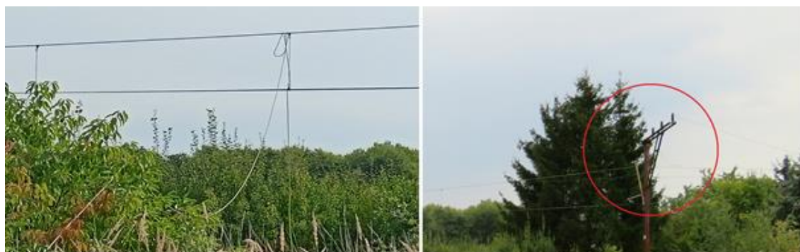
Figure 4. Damaged railway electric traction line [source: Aero Club Zagłębia Miedziowego]
