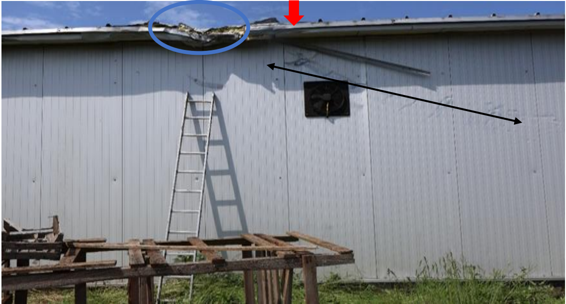
Figure 3. The place of the aeroplane's impact on the building: the main impact on the edge of the roof (blue circle), the impact of the right wing (black line), the impact of the front fuselage (red arrow).
